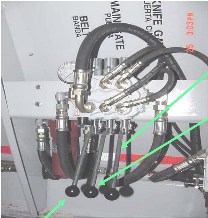
MANUAL VALVE PICTURED
